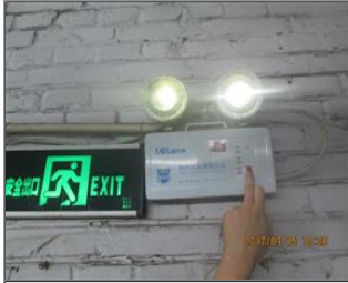
Photo of fire safety equipment Testing emergency light.JPG
