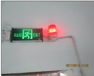
Photo of fire safety equipment Testing fire alarm.JPG
